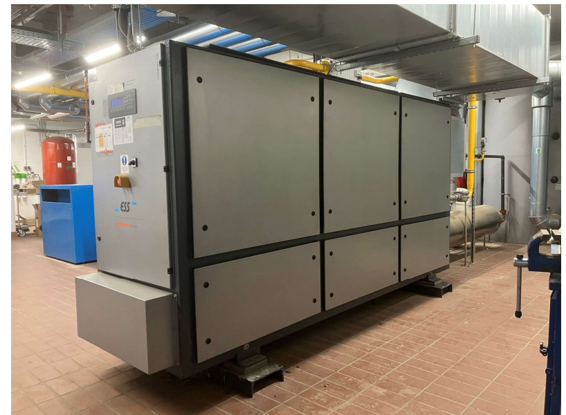
BHKW (207 KW th , Bj. 2012)
