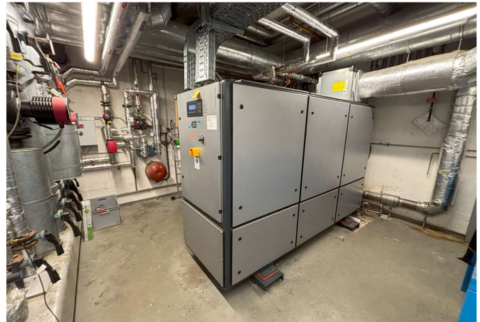
BHKW (81 KW th , Bj. 2015)
